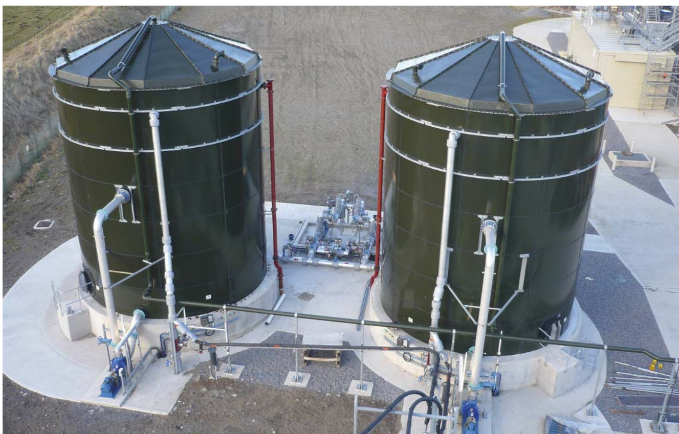
New limed sludge storage tanks
