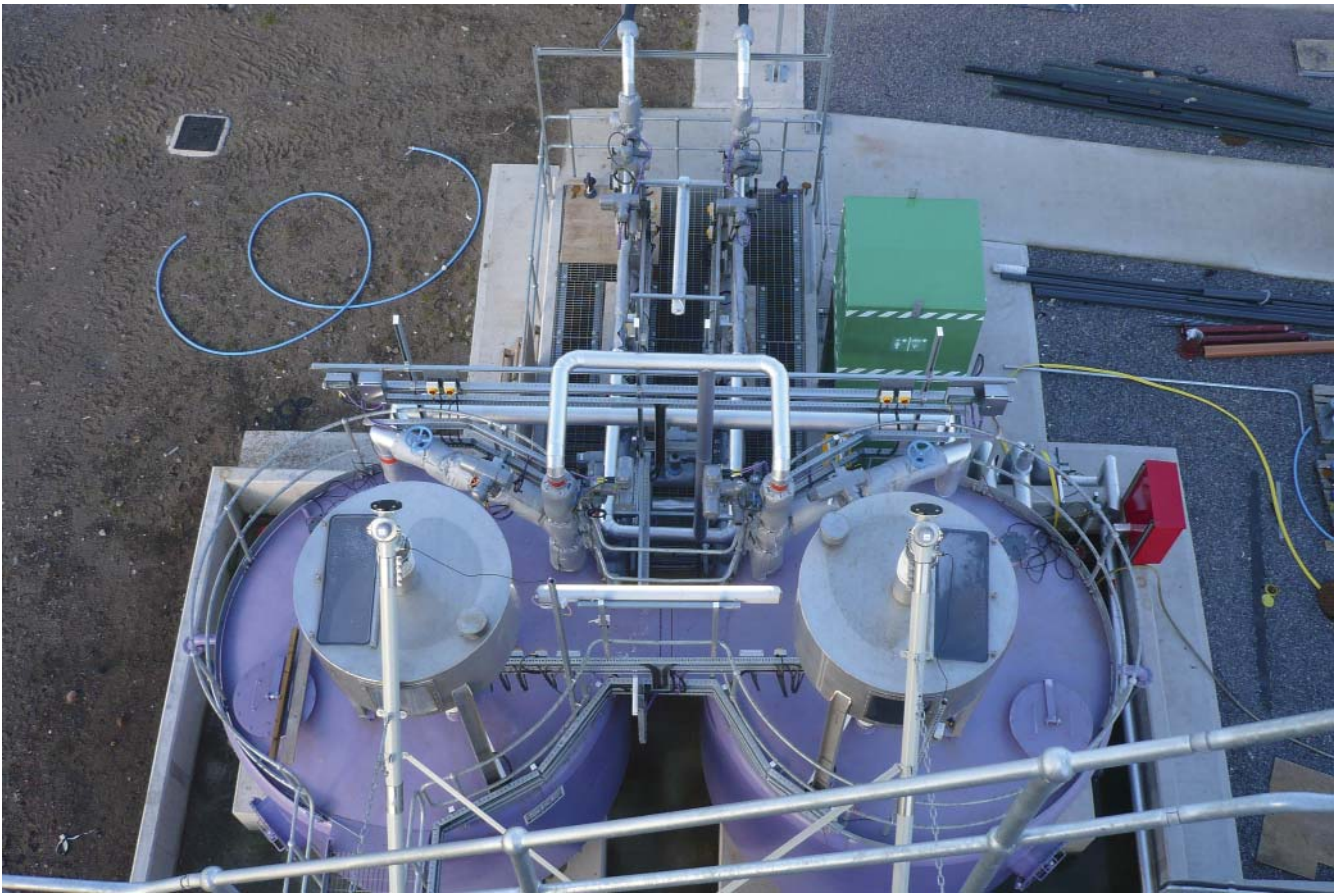
Lime batching and dosing system
