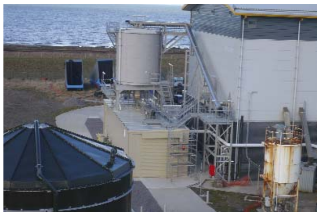
Existing sludge building with new cake silo and loading bay. 1 of 2 new limed sludge tanks in foreground
