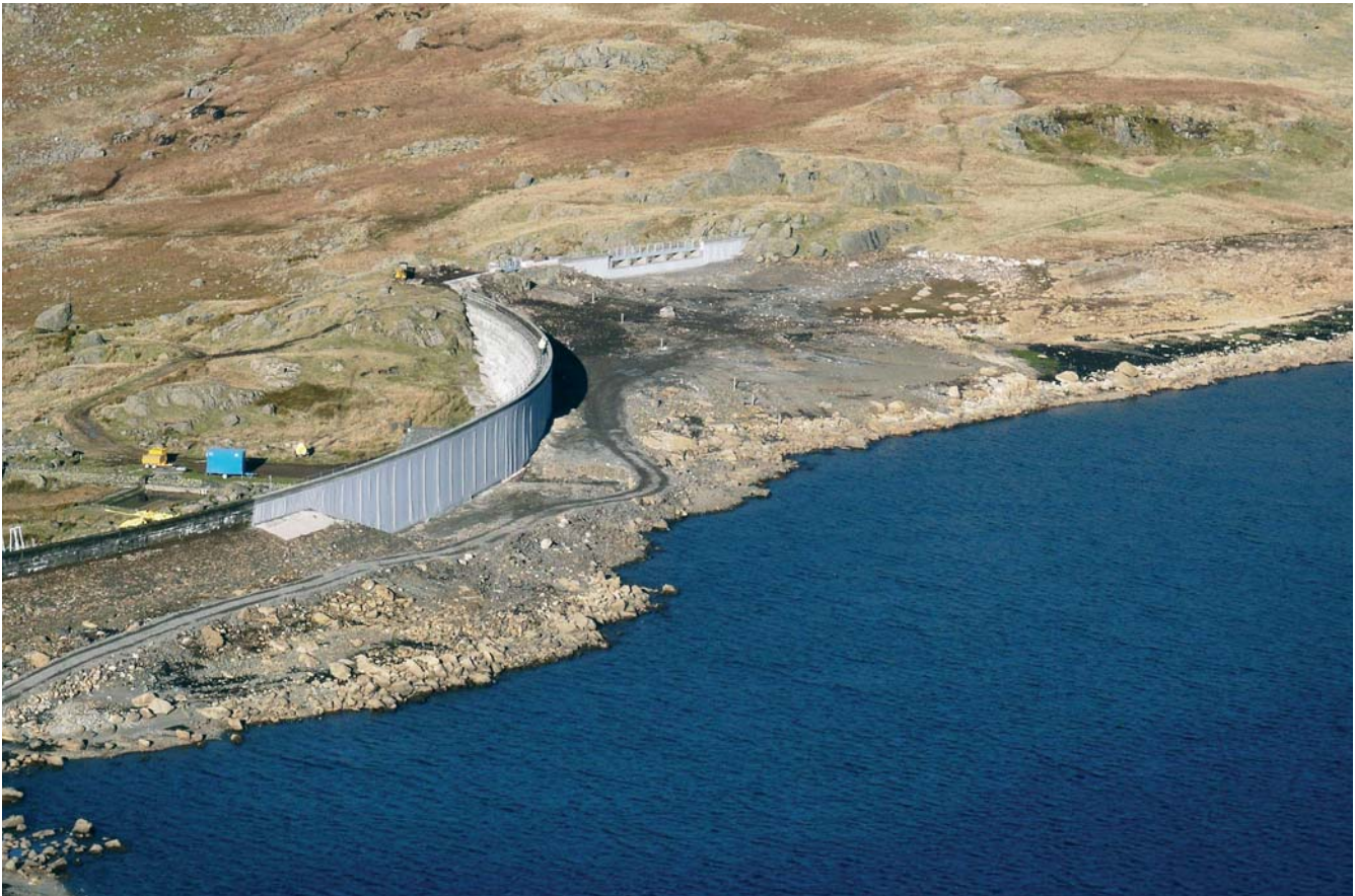
Aerial view, upstream face of concrete dam and auxiliary overflow showing temporary access and Carpi Membrane Courtesy of Eric Wright Civil Engineering Ltd and MWH
