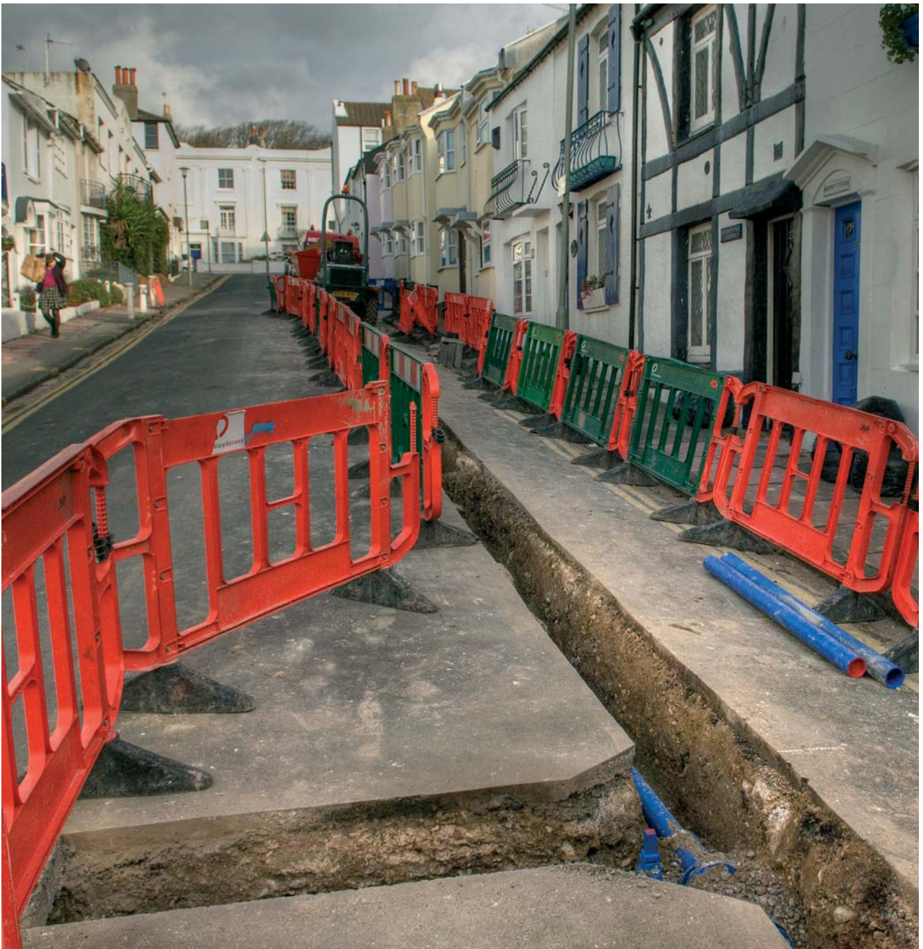
Photograph shows a new pipe having been laid in Brighton City Centre
