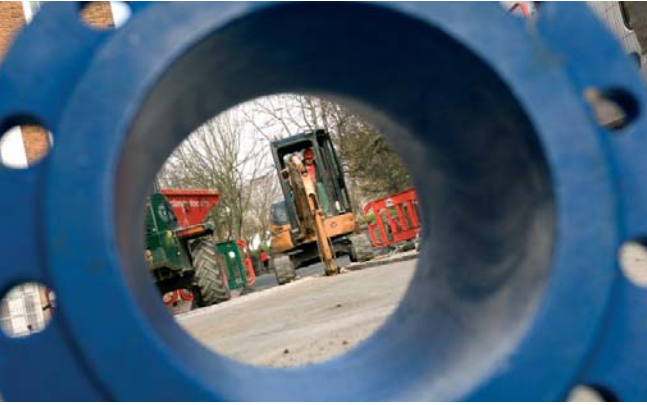
Clancy Docwra work on the Brighton Water Mains Replacement on Dyke Road, Brighton City Centre Courtesy of Southern Water
