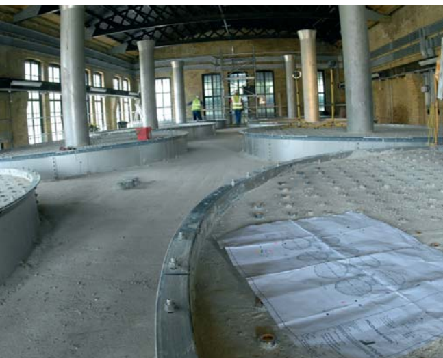
Rapid Gravity Filters under construction Photograph by Ady Kerry, courtesy of South East Water
