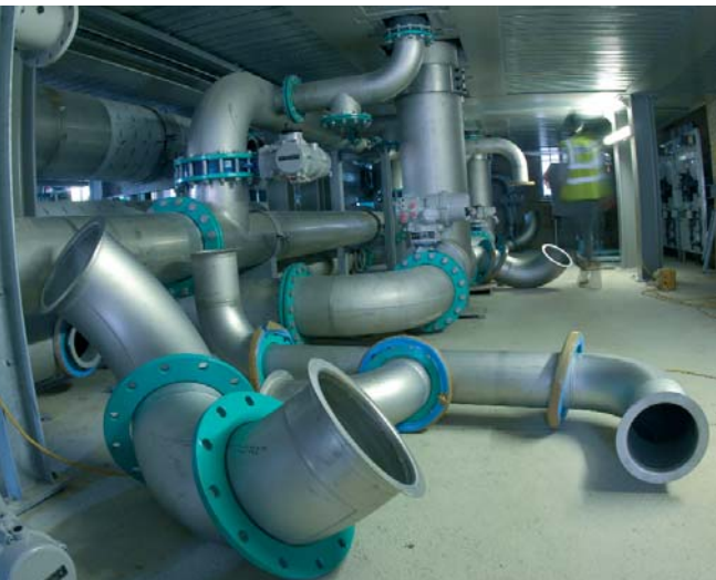
Associated Rapid Gravity Filter pipework under construction Photograph by Ady Kerry, courtesy of South East Water
