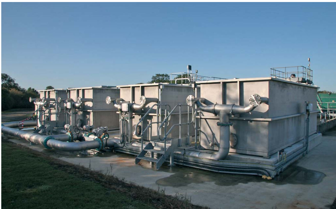
HSAF Solids Filter built for Yorkshire Water for a P removal project
