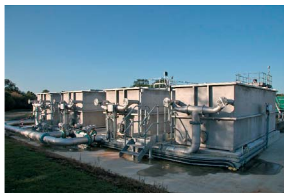
HSAF Solids Filter built for Yorkshire Water for a P removal project
