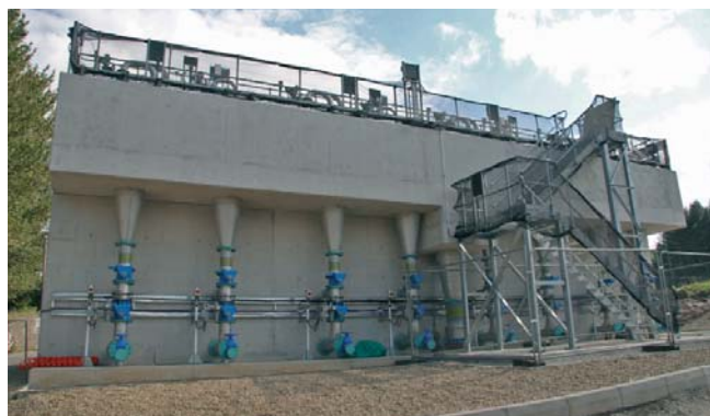
Large Scale HSAF delivering consent compliance at 1 mg ammonia/l on a 95%ile basis, whilst using only one third of the power of alternative SAF technology, built for United Utilities
