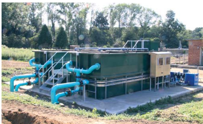
HSAF Solids Filter built for Anglian Water as part of a P removal project
