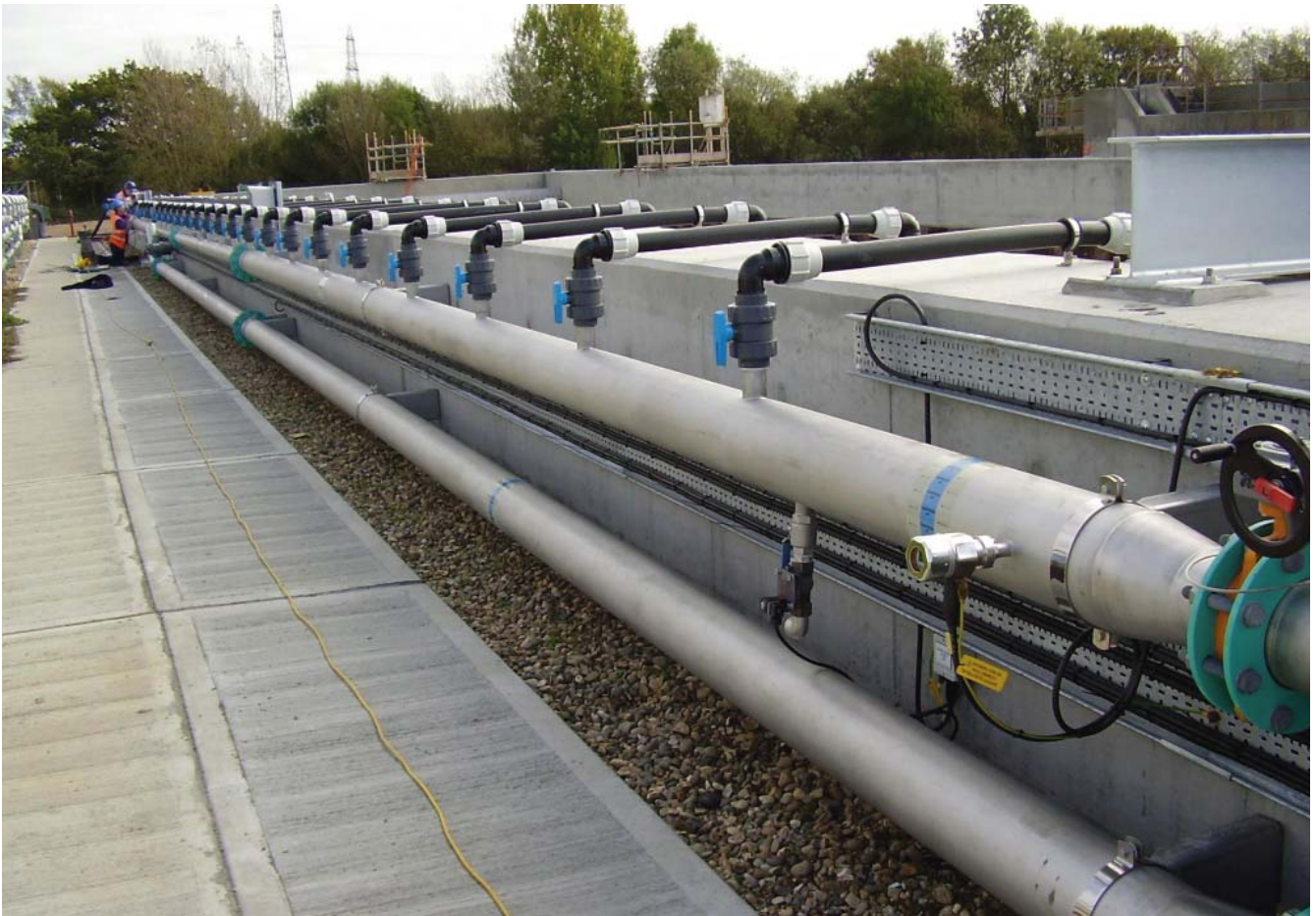
Aeration lane air pipework
