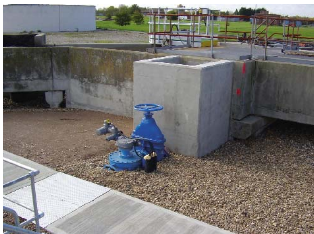
Flow split diversion chamber and modulating valve Courtesy of the @one Alliance
