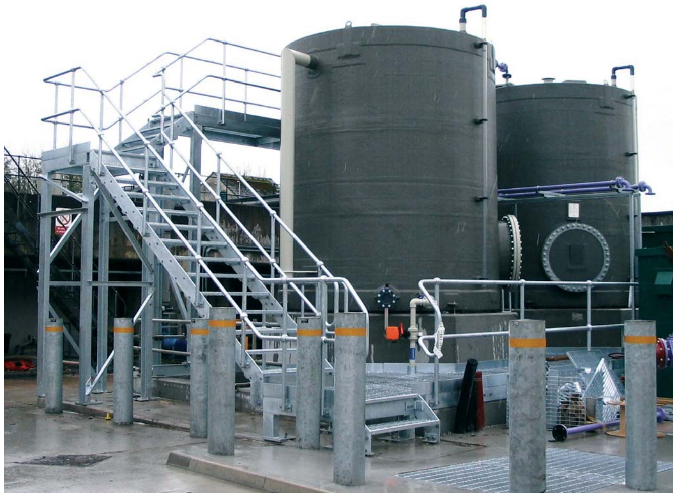
New ferric sulphate bulk storage tanks
