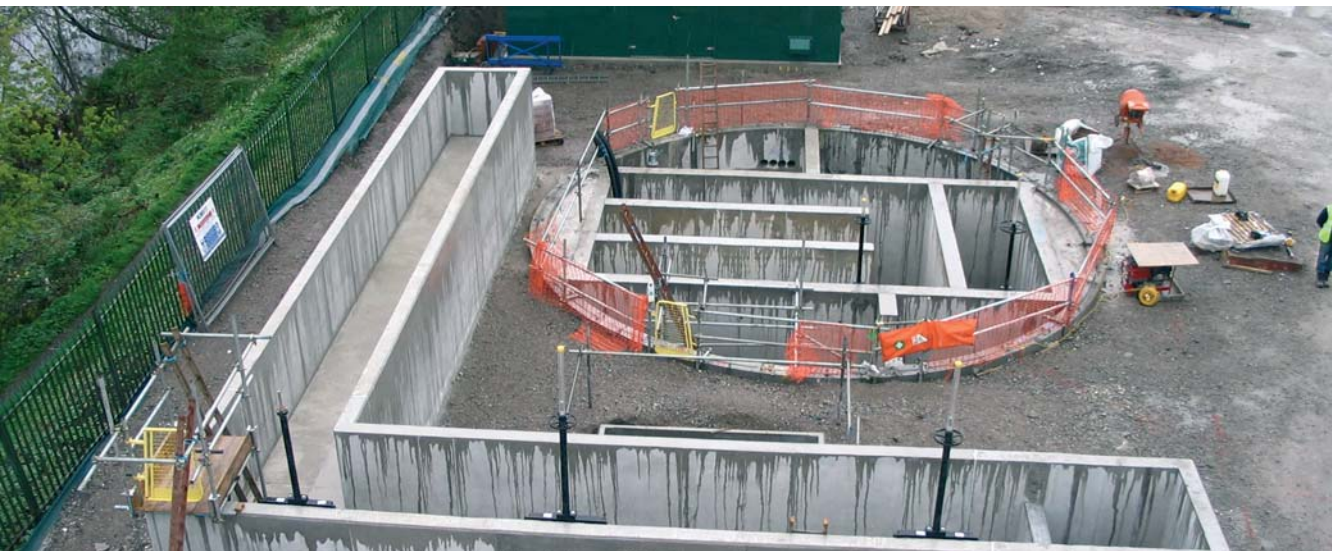
From Top, Interstage Pumping station MCC Kiosk, Interstage Pumping Station awaiting pumps, Feed channel and Disc Filters
