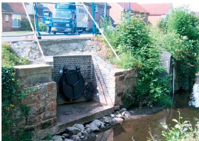
New CSO Outfall at Finham Brook Courtesy of Severn Trent Water Ltd
