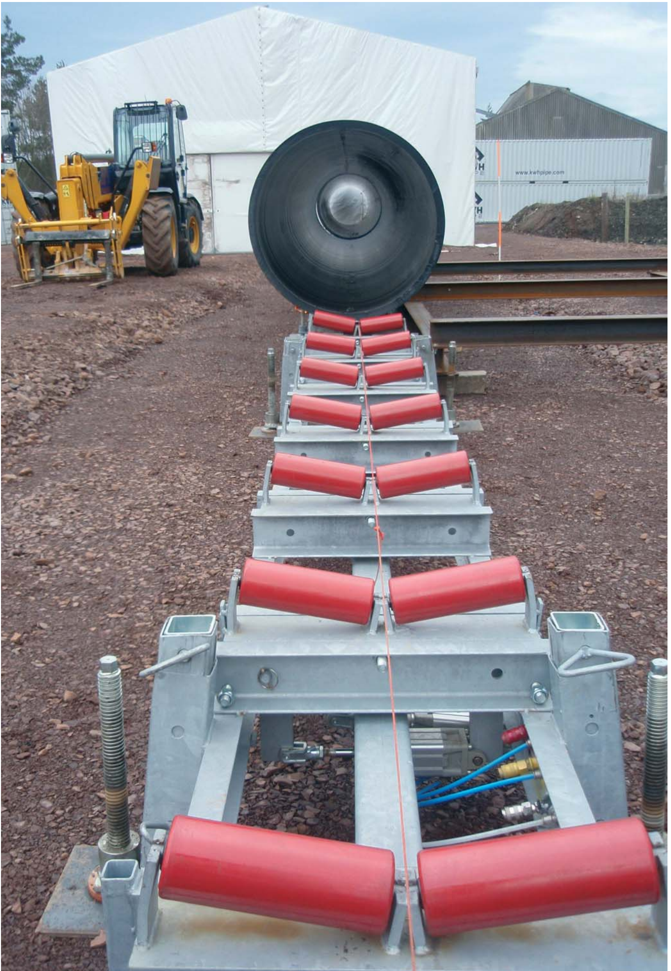
Glencorse Pipe Production plant
