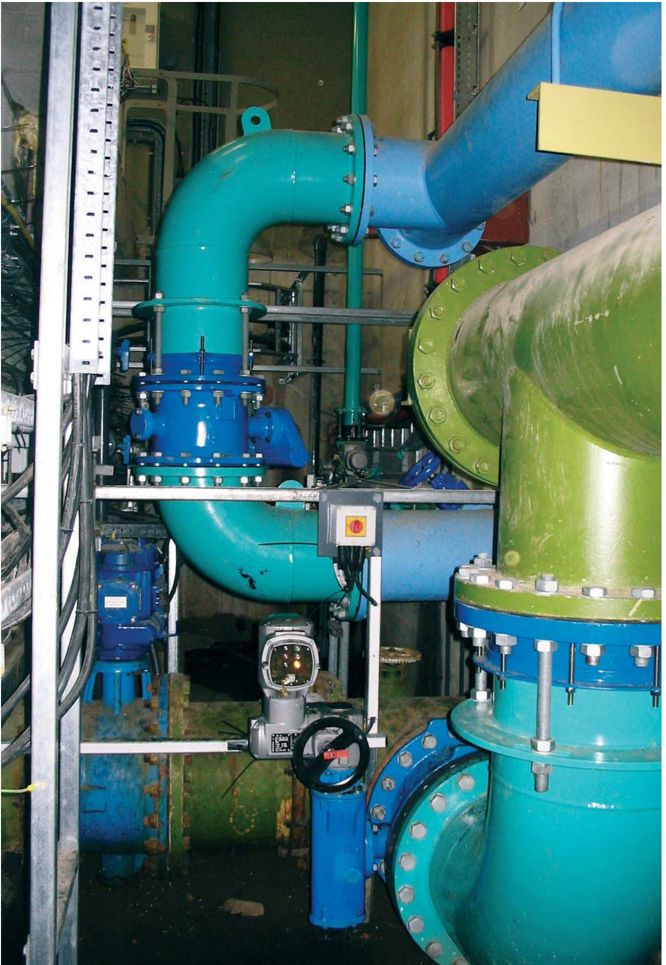
New backwash and air scour Valves
