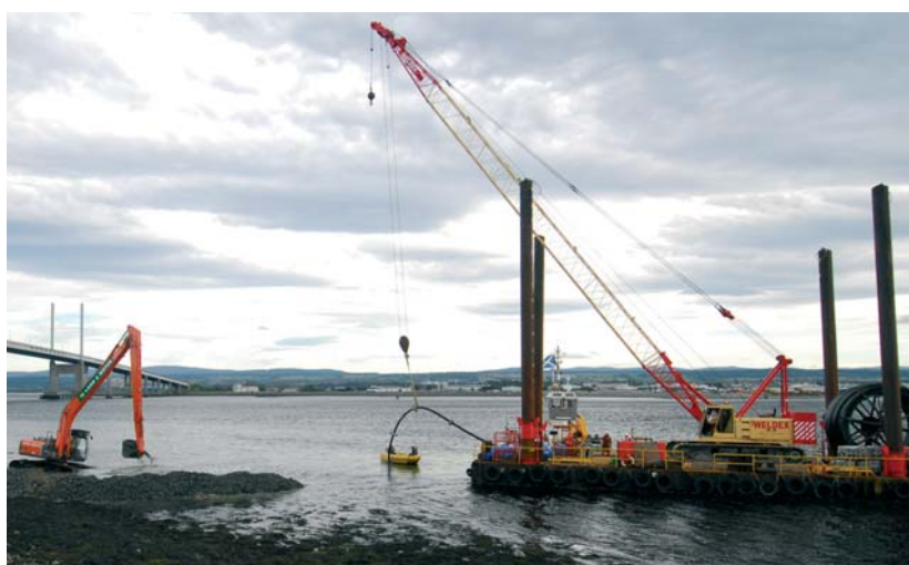
Commercial Marine & Piling installing, trenching and backfilling sewage pumping main across the Beaully Firth in water currents up to 7 knots. 2007
