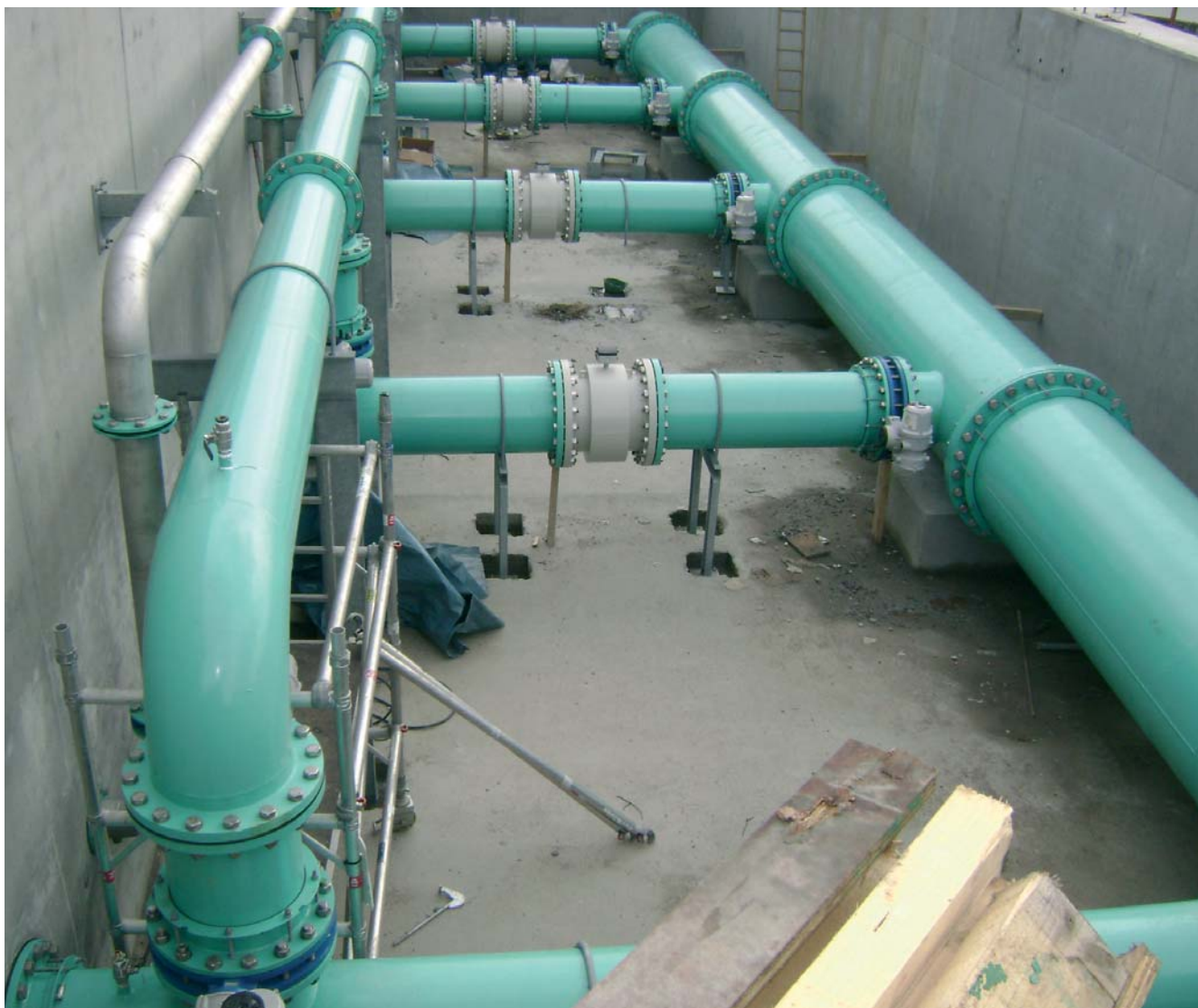
RGF Pipe gallery
