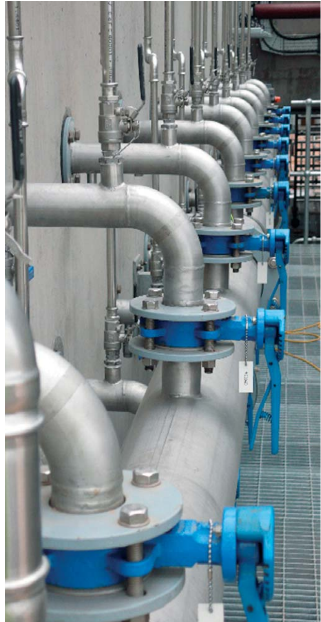
Final effluent (permeate) gallery prior to pipe insulation being fitted photo courtesy Black & Veatch Water Europe
