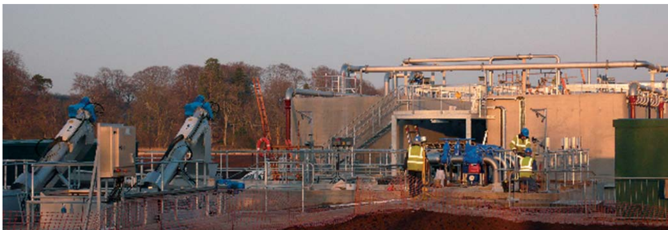
Screens in the foreground & MBR cells in background
