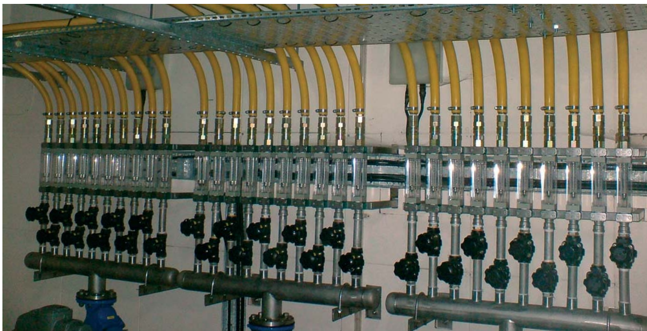
Upper Tamar Lake - Air delivery manifold
