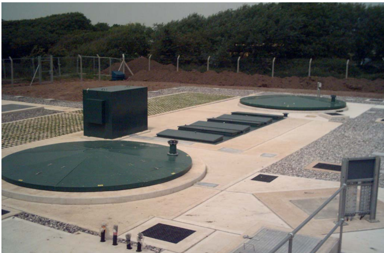
Kilve STW Secondary treatment provided
