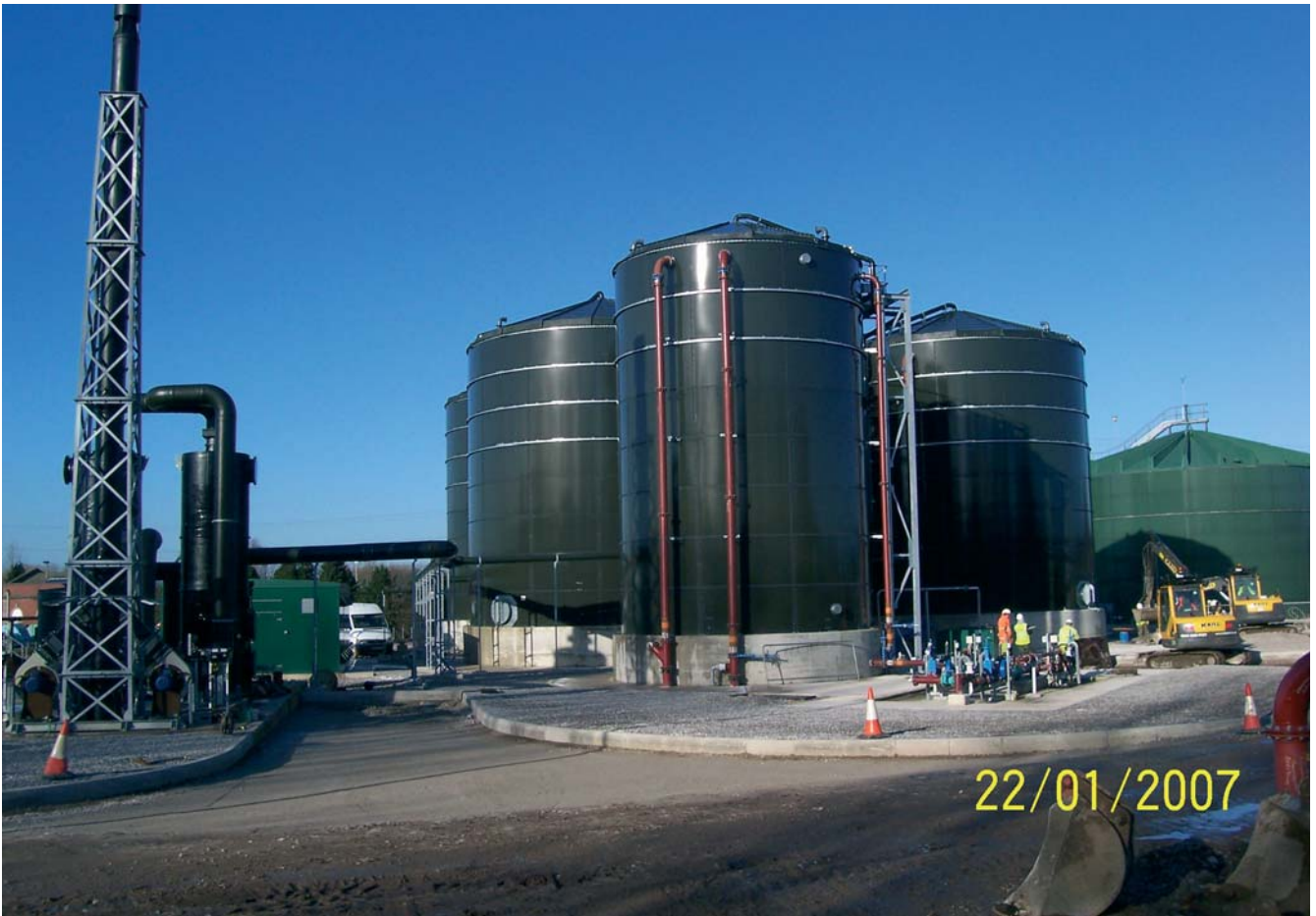
Stockport WwTW: Consolodation tanks at sludge area
