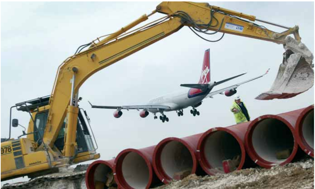
Working safely with minimum disruption to Manston Airport to bring cleaner seas to Margate & Broadstairs
