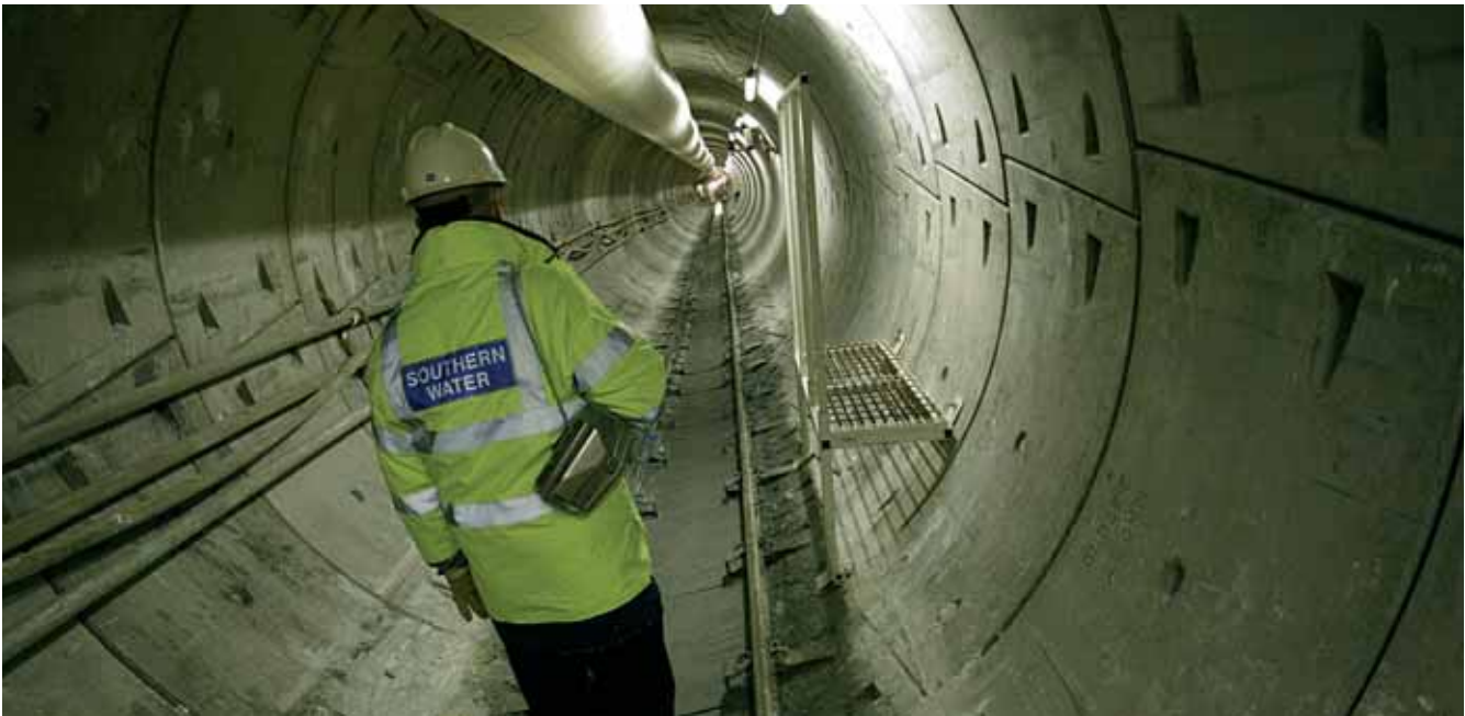
Margate Tunnel: Light at the end of the tunnel as work continues on 1380m long tunnel
