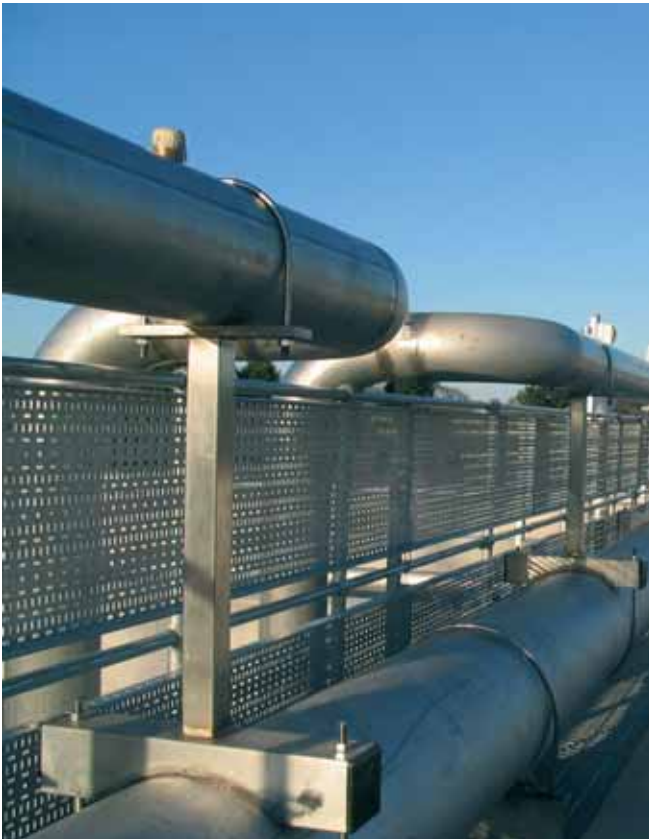
ASP Blower air main
