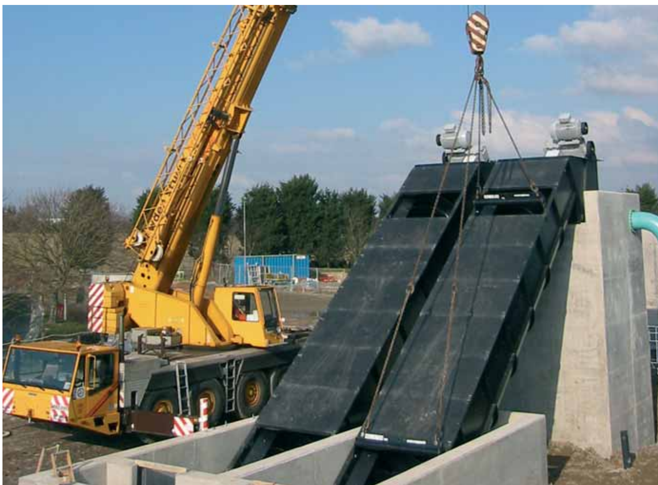
Monkmoor STW: Spaans screw pump installation
