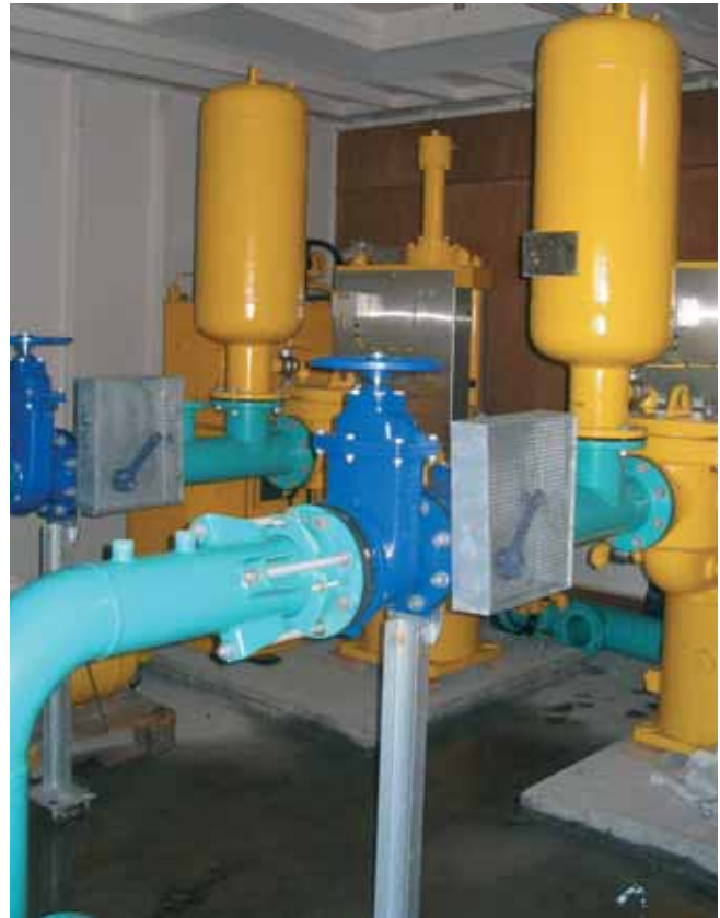
Sludge Ram Pumps
