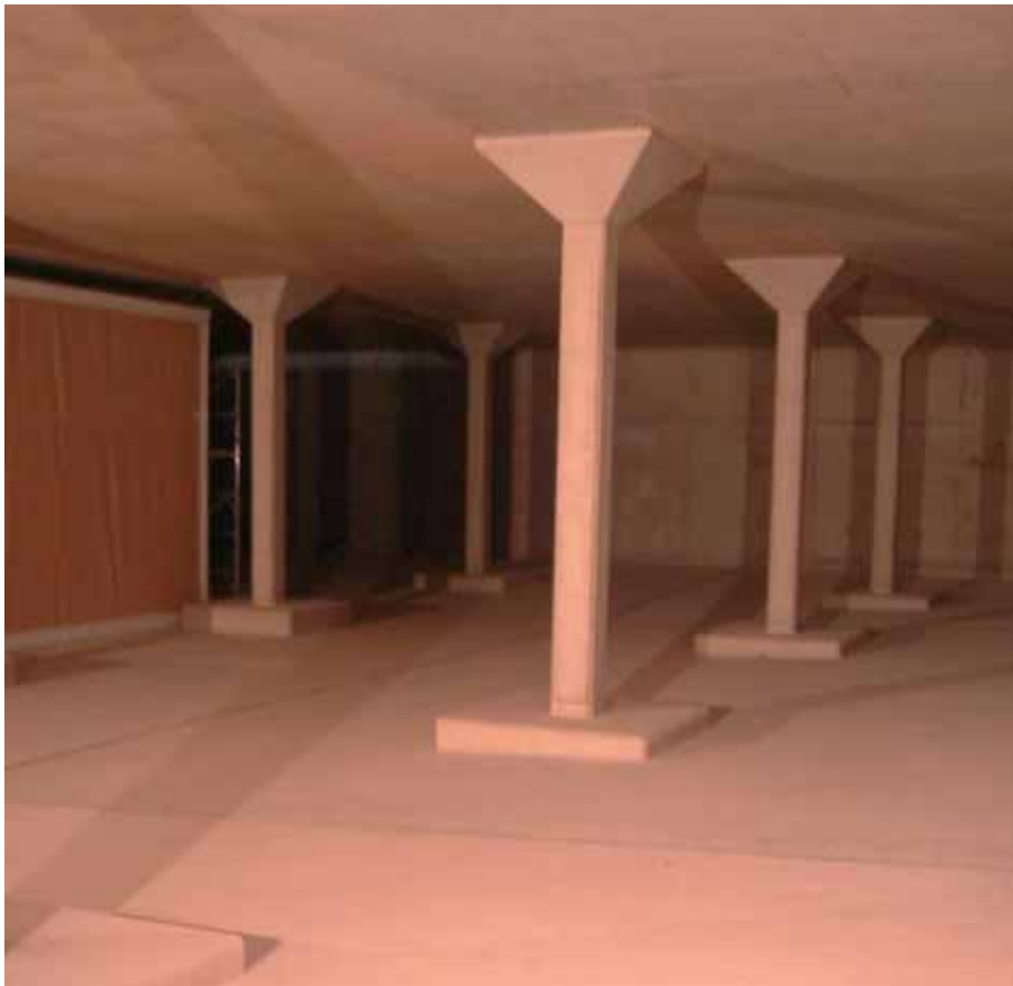
Stanborough: Inside the service reservoir
