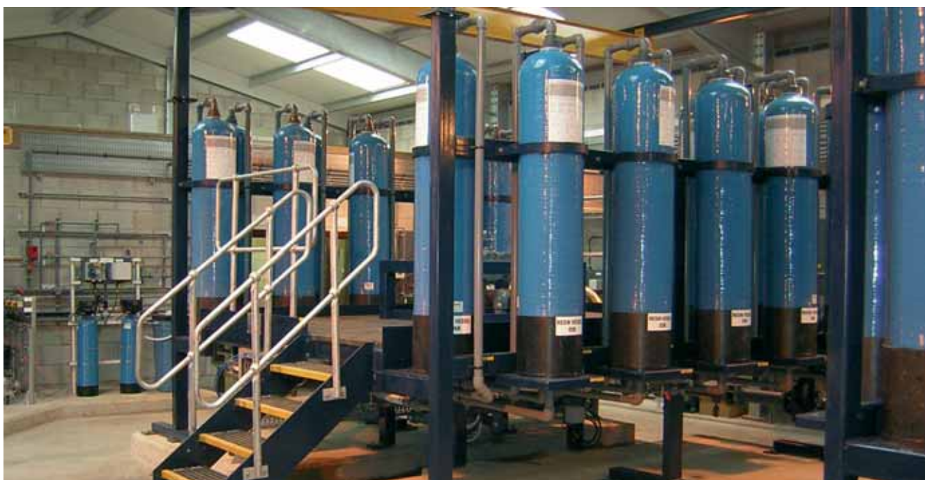
Lyng Forge: Nitrate removal skid
