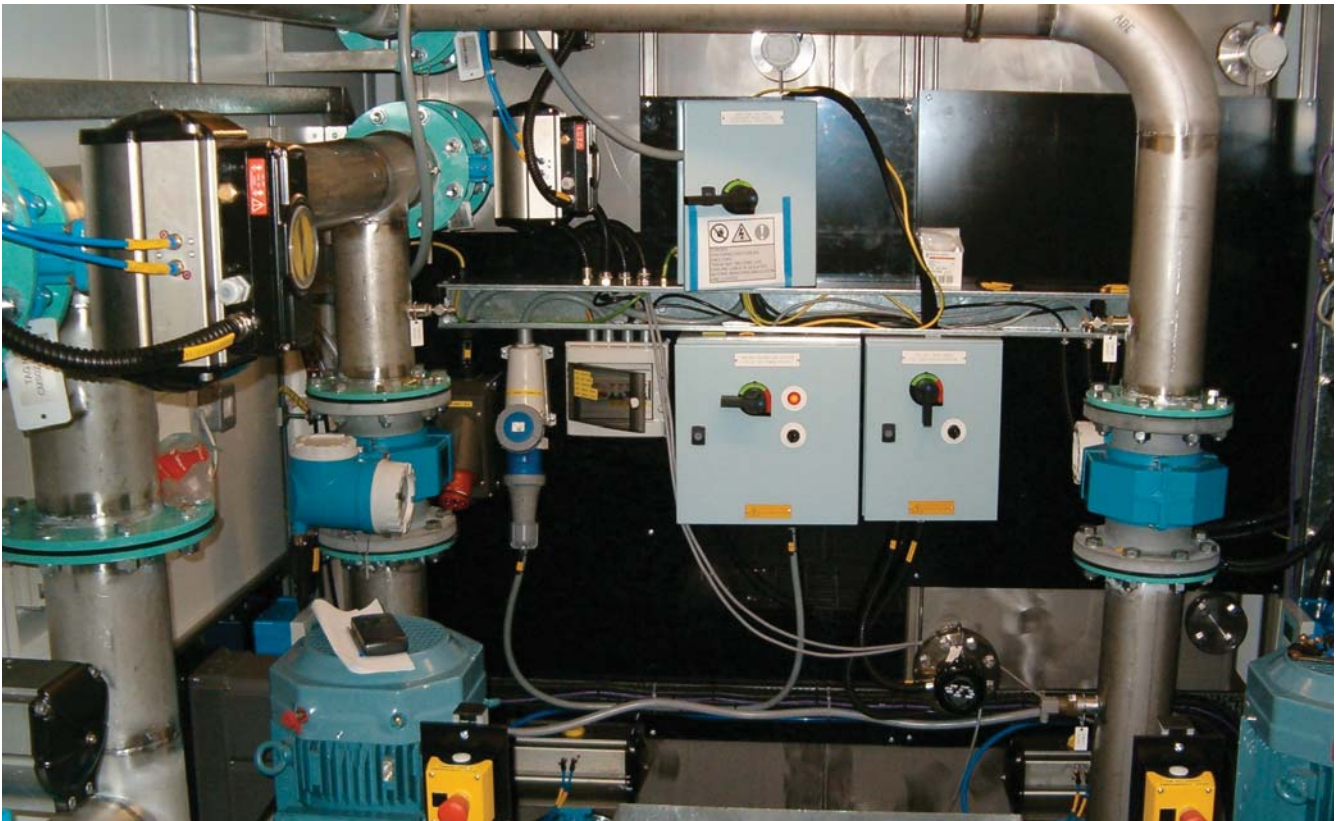
Inside a container the Emergency Packaged Water Treatment plant being fitted out
