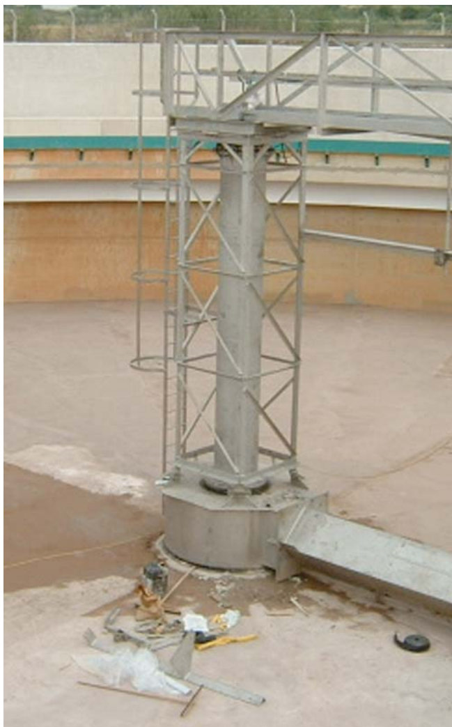
Warrington Rim Flo clarifier tow bro arm used for final screeding of base slab
