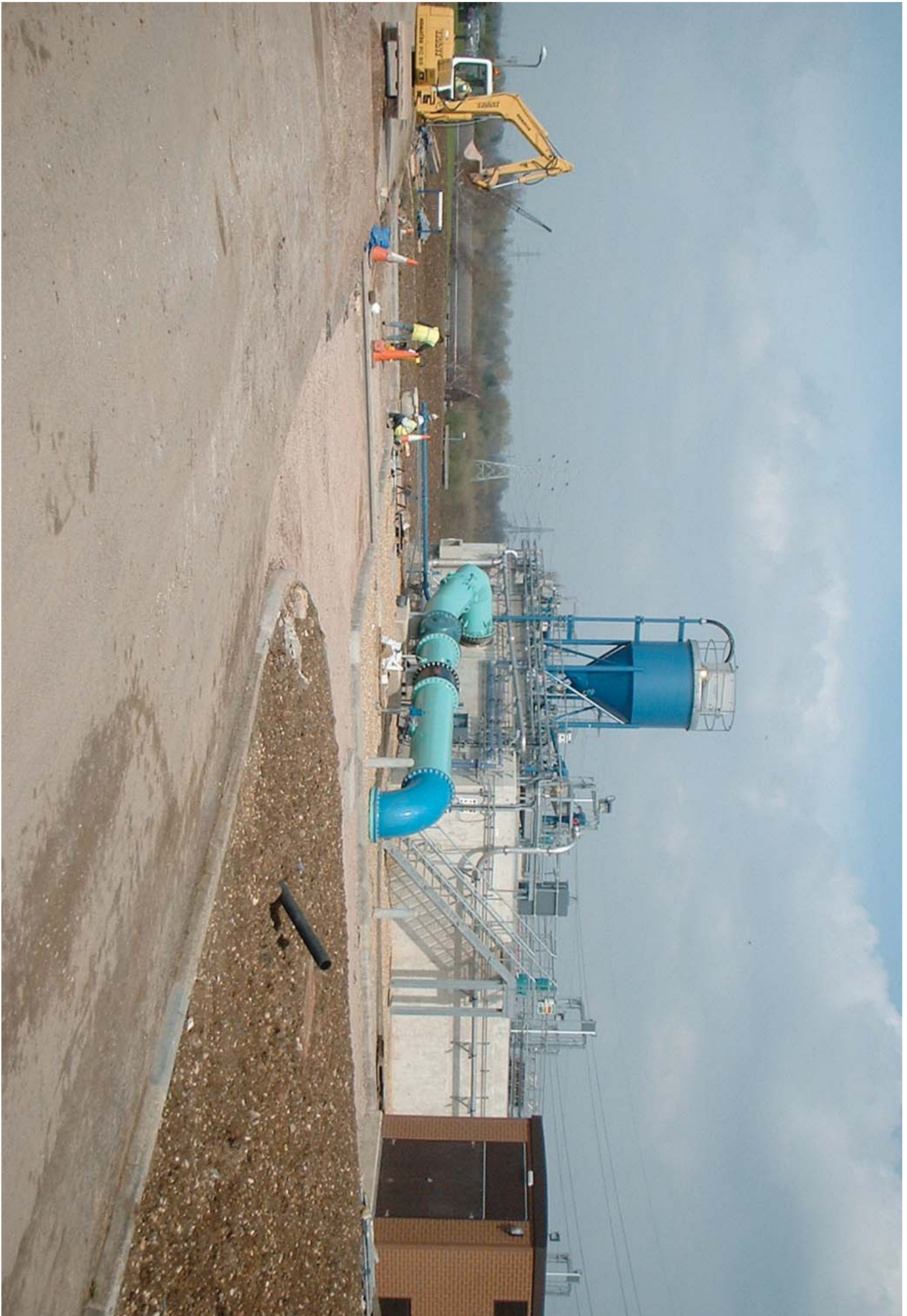
Iver WTW: Existing pulsator clarifiers and location of third stream
