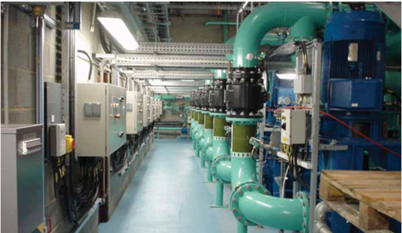
Chertsey WTW: Main membrane filtrate pumps & pipework
