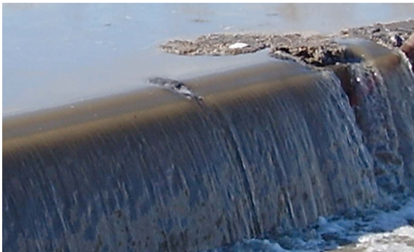
Trent Vale PS: Water starting to weir over the cut out sections
