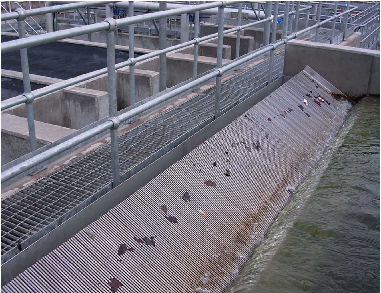
Workshop STW: Manual screen on inlet to protect proprietary T blocks
