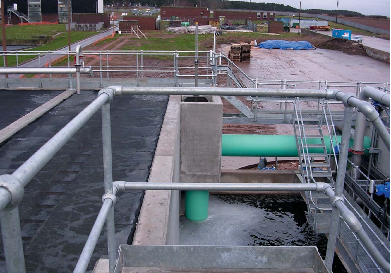
Worksop STW: Outlet from the NSAF
