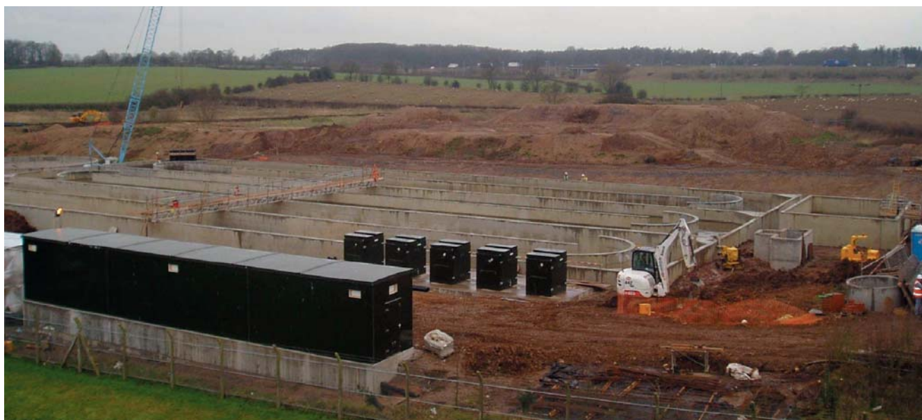
Packington STW: New oxidation ditches, MCC & blowers.
