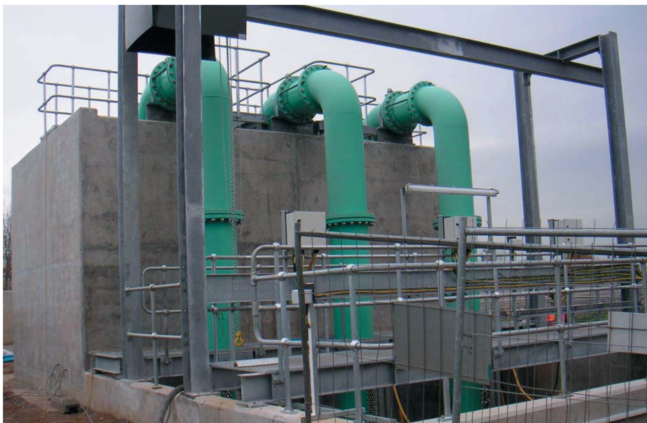
Hartshill: New intermediate pumping station allocates flow between new & existing works
