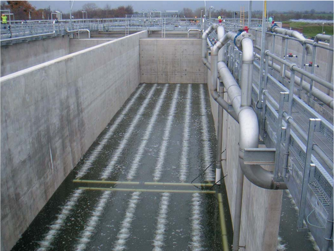
Hartshill: ASP2 aeration lanes, fitted with diffuser grids of varying densities.
