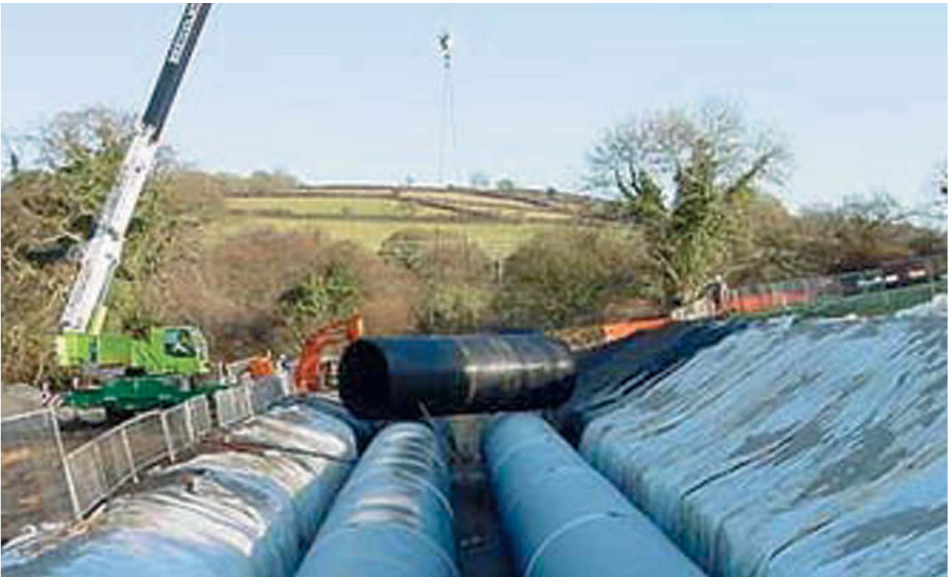
Tamerton Foliot, Devon: Removal of a DG5 flooding problem at Hayesend Farm
