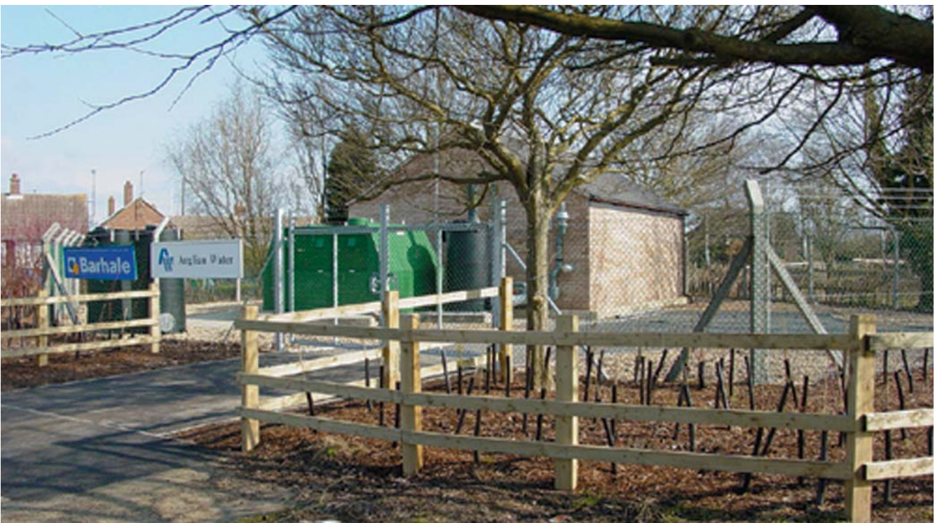
Upwell & Outwell: One of the vacuum stations in the UK's largest vacuum sewerage system
