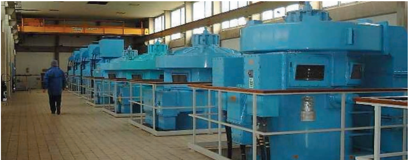
Franklaw WTW - Pumps in treated water house
